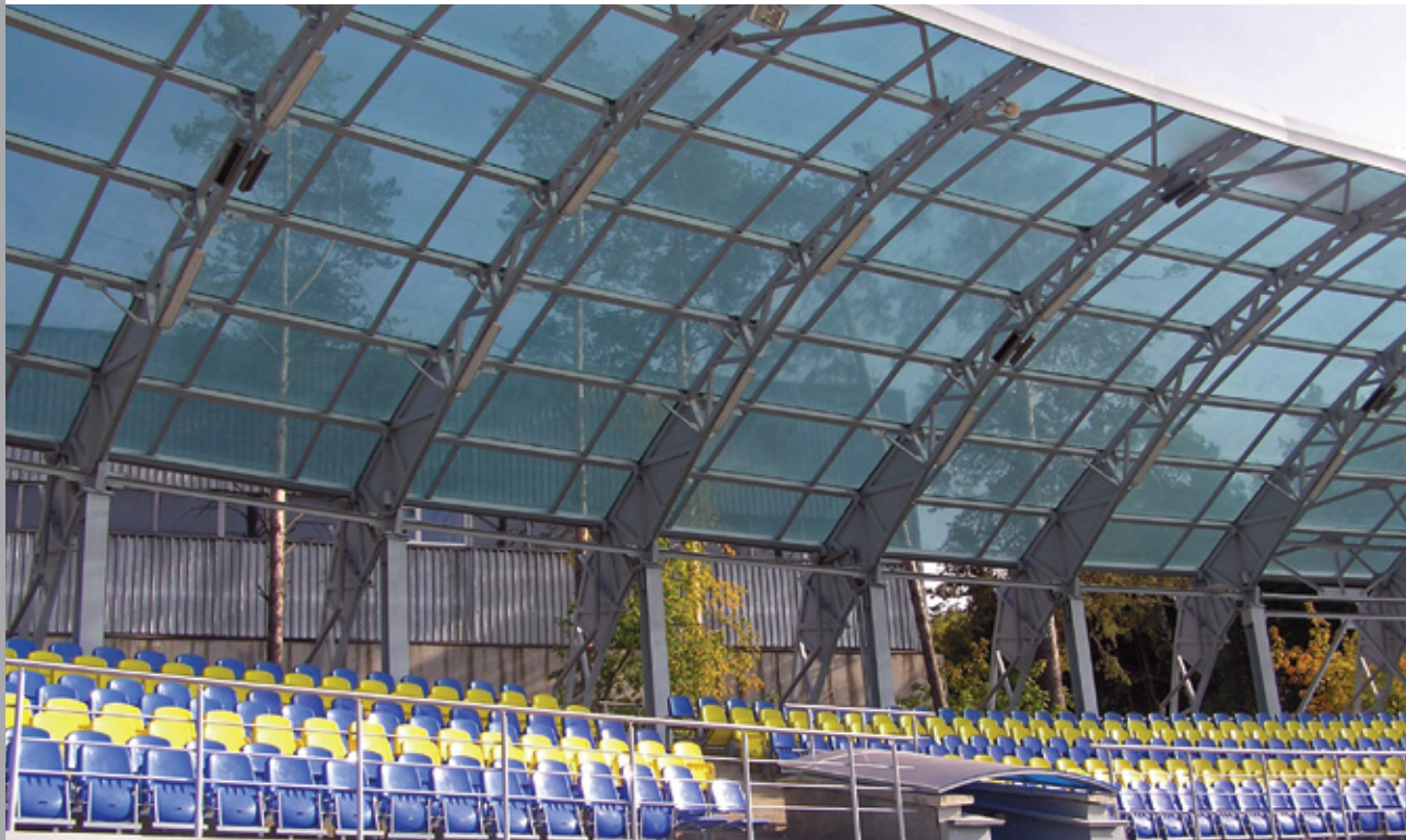
PALSUN 10mm Solar Olympic sheets installed at the "Electron" stadium in Novosibirsk, Russia (See article inside).
